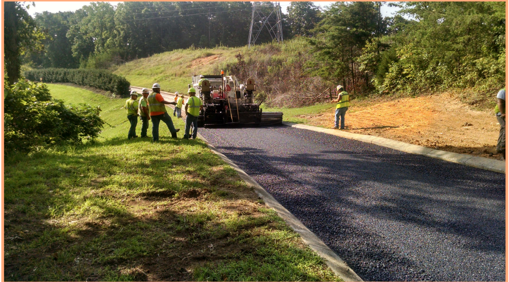
Repair of Ladd Landing Boulevard is complete following a 12-inch waterline leak that “blew out” the roadway.
