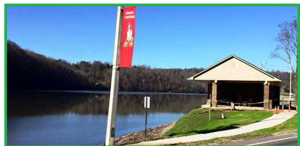
Work on the new pavilion at the Gravel Pit is coming right along! Beautiful addition to the Watts Bar lakefront!
