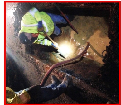
Sewer break on Circle Drive
